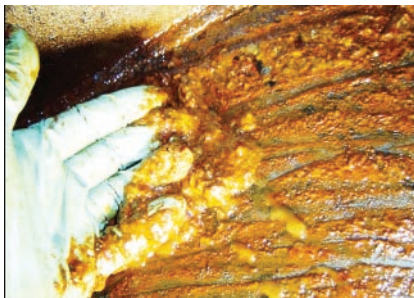
2. Sludge found in this main reduction gear system was no surprise, because oil analysis of samples had revealed high water contamination
