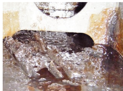
5. Gels or slime may develop from reactions between incompatible fluids or from certain contaminants. Here's a gel layer that formed in a contaminated system that uses phosphate ester as a hydraulic control fluid. Sample acid number was greater than 4.0
