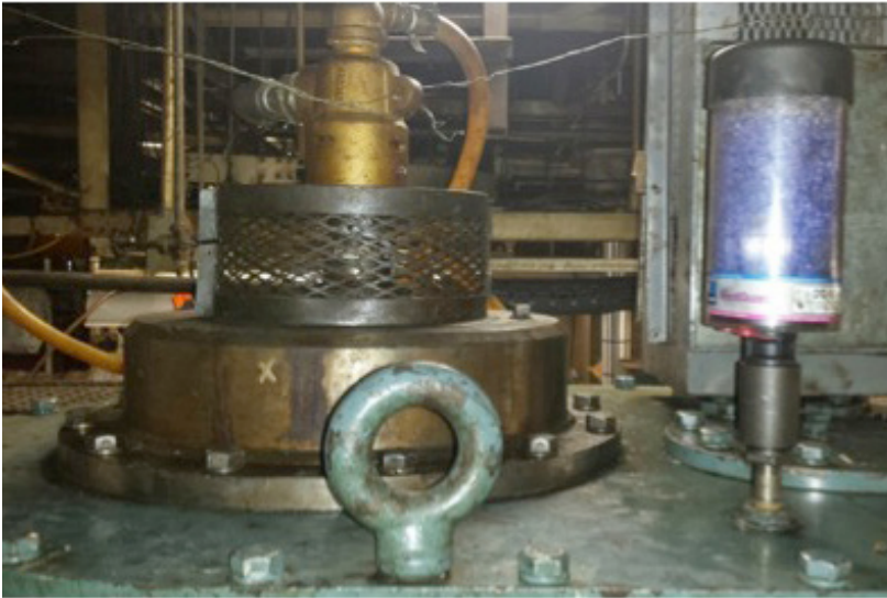
Figure 2 - Side view of the Autoclave gearbox rotary joint
